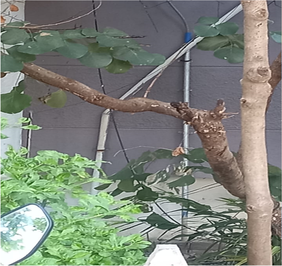
Pipe Line For Water Collection
